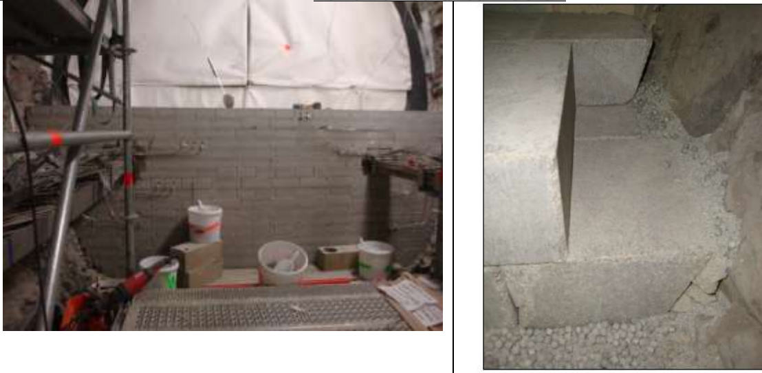
Figure 8 Installation of bentonite core, wall made with bricks, pellets/powder mixture between claystone and bentonite bricks. Background: hydration membrane
